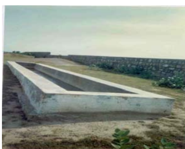
WATER-TROUGH & BOUNDARY-WALL AT ONE OF THE FAIR-SITES CONSTRUCTED UNDER A. D. P.
